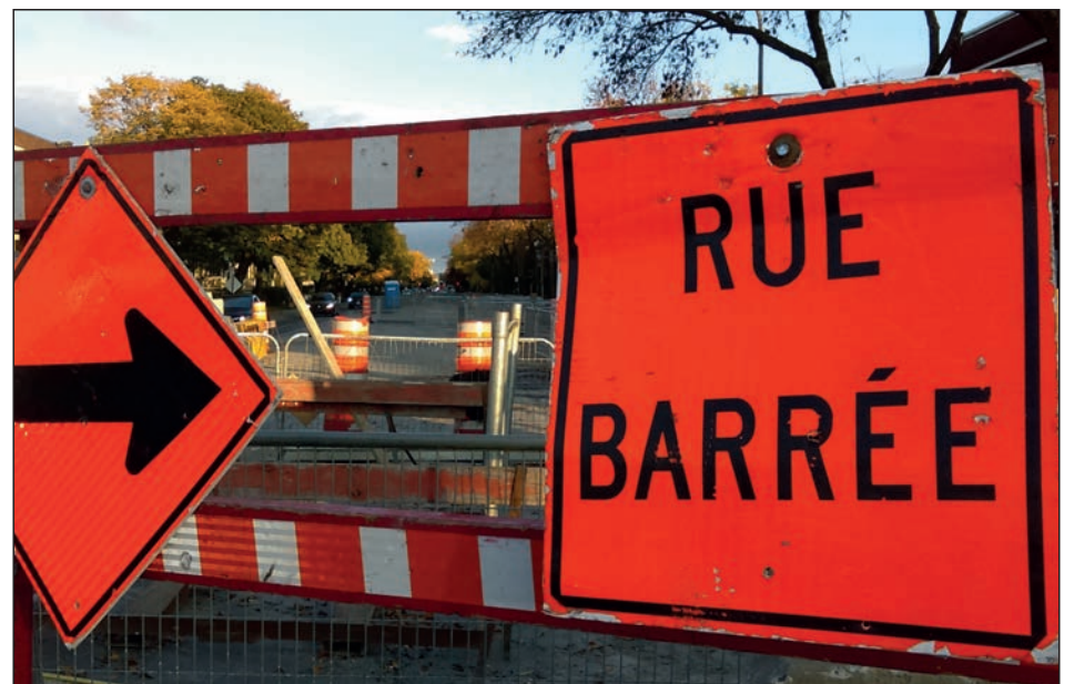
A massive gash in the street runs for many blocks—as of 4:30pm on Monday this week, work had already ceased ... who knows how long this project will last, locals lament
