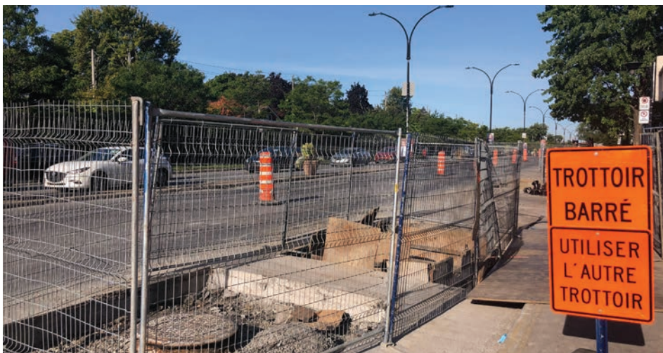
The refurbishment of underground infrastructure on De L'Acadie Boulevard is set to wrap up on Oct. 29. Photo: Matias Brunet-Kirk - NEWSFIRST
